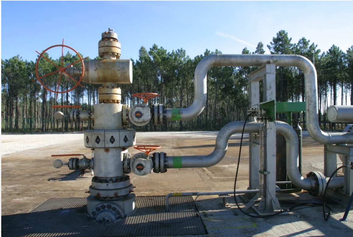
Solution Mining Process – Leaching Wellhead
